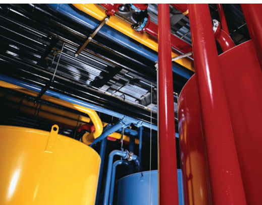
Compressed Air Systems
